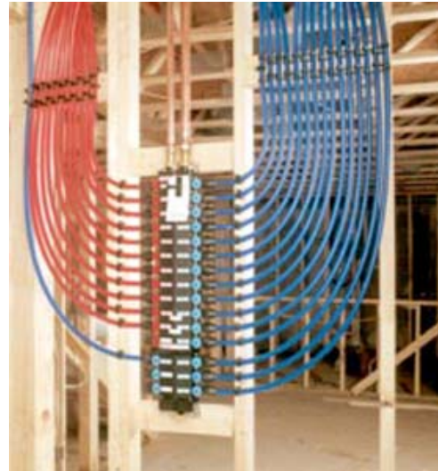
Figure 20 – PEX tubing and remote manifold.
